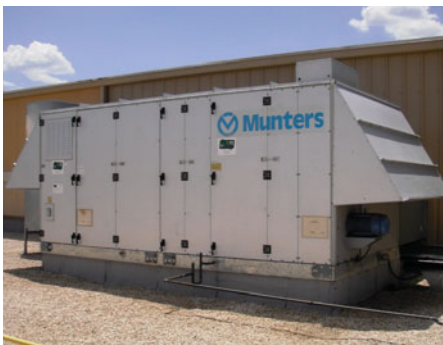
The FreeDry™ unit on the roof of the Chaparral Ice Rink.
