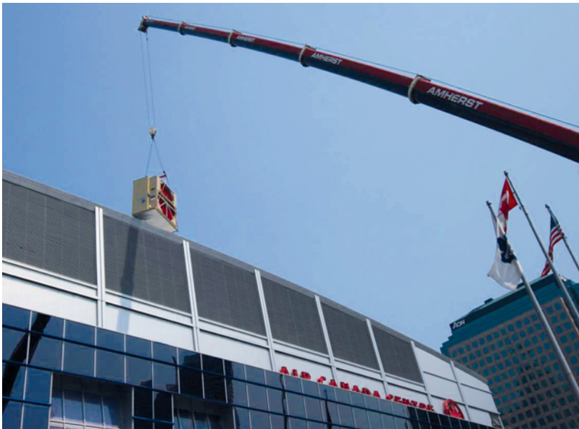
In the summer of 2007, two Munters dehumidifiers were installed at the Air Canada Centre to successfully treat the air to meet NHL ventilation requirements.
